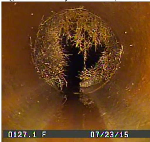
Figure 4: Sanitary Sewer Line, Tree Root Intrusion
